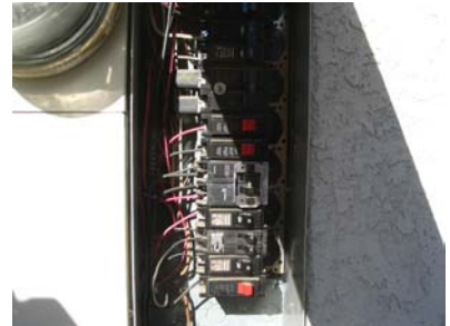
Electrical panel in good order
