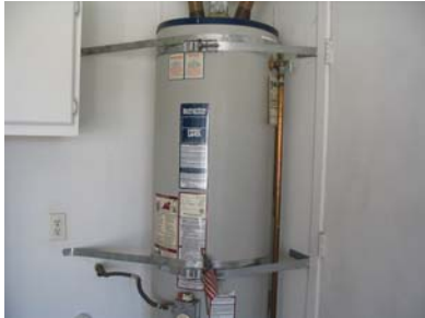
Water heater properly strapped
